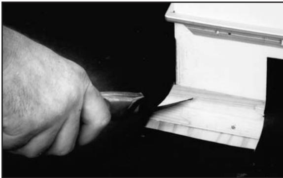
Fig. 104. Insert knife blade into cove fillet miter and extend cut to subfloor.
